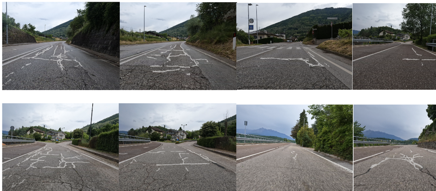
Examples of road surface deterioration (pavement cracks) identified by the Edilpavimentazioni survey system
